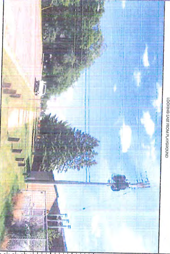
POWER POLE #19AA13 LOOKING EAST ALONG COLEMAN STREET
